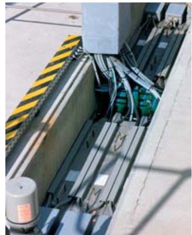
TAK-Anlage in Tywyn, Wales
